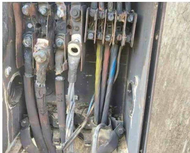
Aging Cable Image
